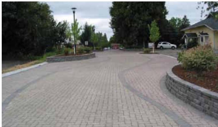
Gresham, Oregon, engineered a PICP street with an open-graded aggregate base and sub-base to accept vehicular traffic while capturing and treating rainwater.
