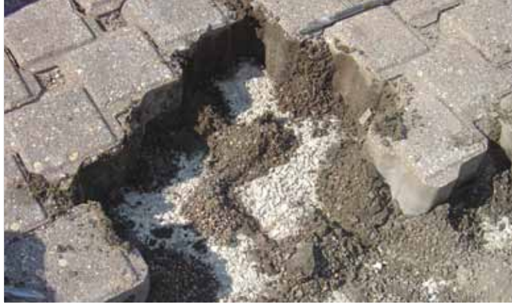
This profile of a clogged paver demonstrates sediment travel path and principle of an infiltration trench that collects pollutants and improves water quality.
